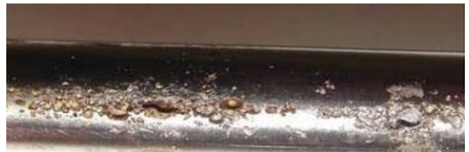
Figure 1: Pitting corrosion on Stainless Steel
